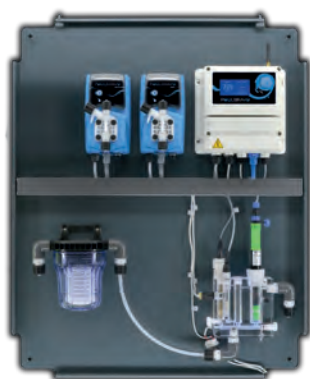
POOL BRAVO + ACID PUMP + CHLORINE PUMP
